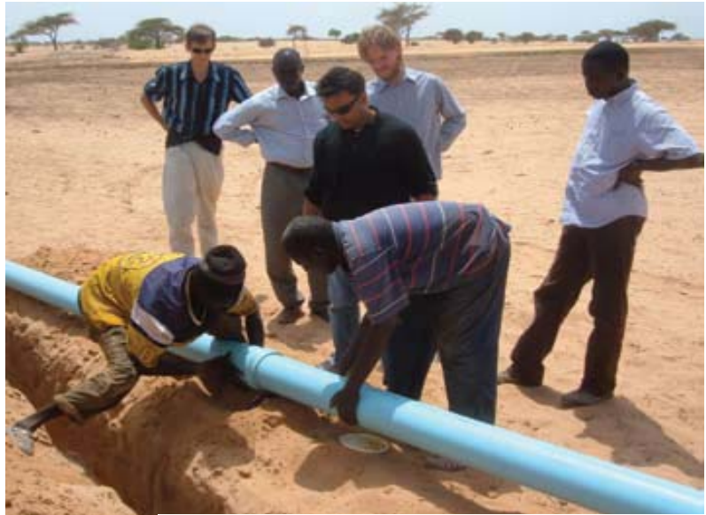
Installation of pipe donated by JM Eagle for the water distribution system in Potou, Senegal
